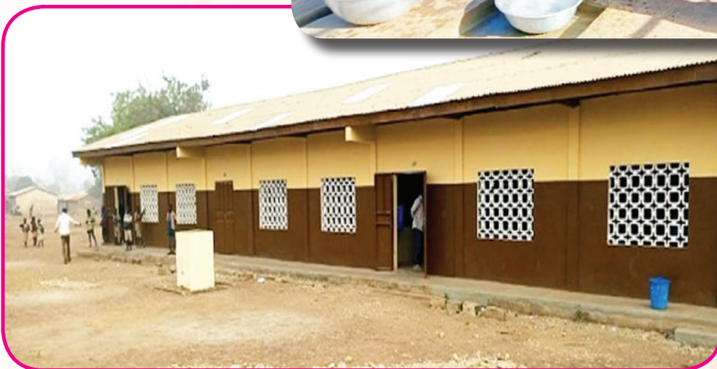
Renovation of a three-class module by the AGIR-Benin project at the EPP Sayakrou commune of Pehunco
